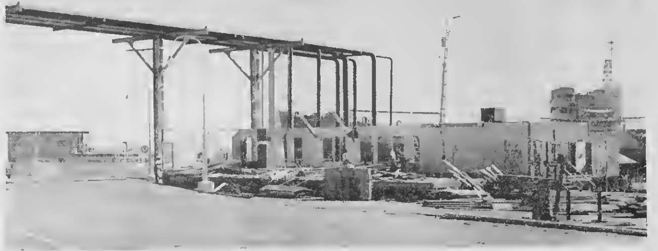
Timbers that rank as "ancient" by refinery standards were being pulled apart this month as the old EIG building was torn down following the group's move to new quarters near the Postoffice. Dating from 1928, the structure was one of the
